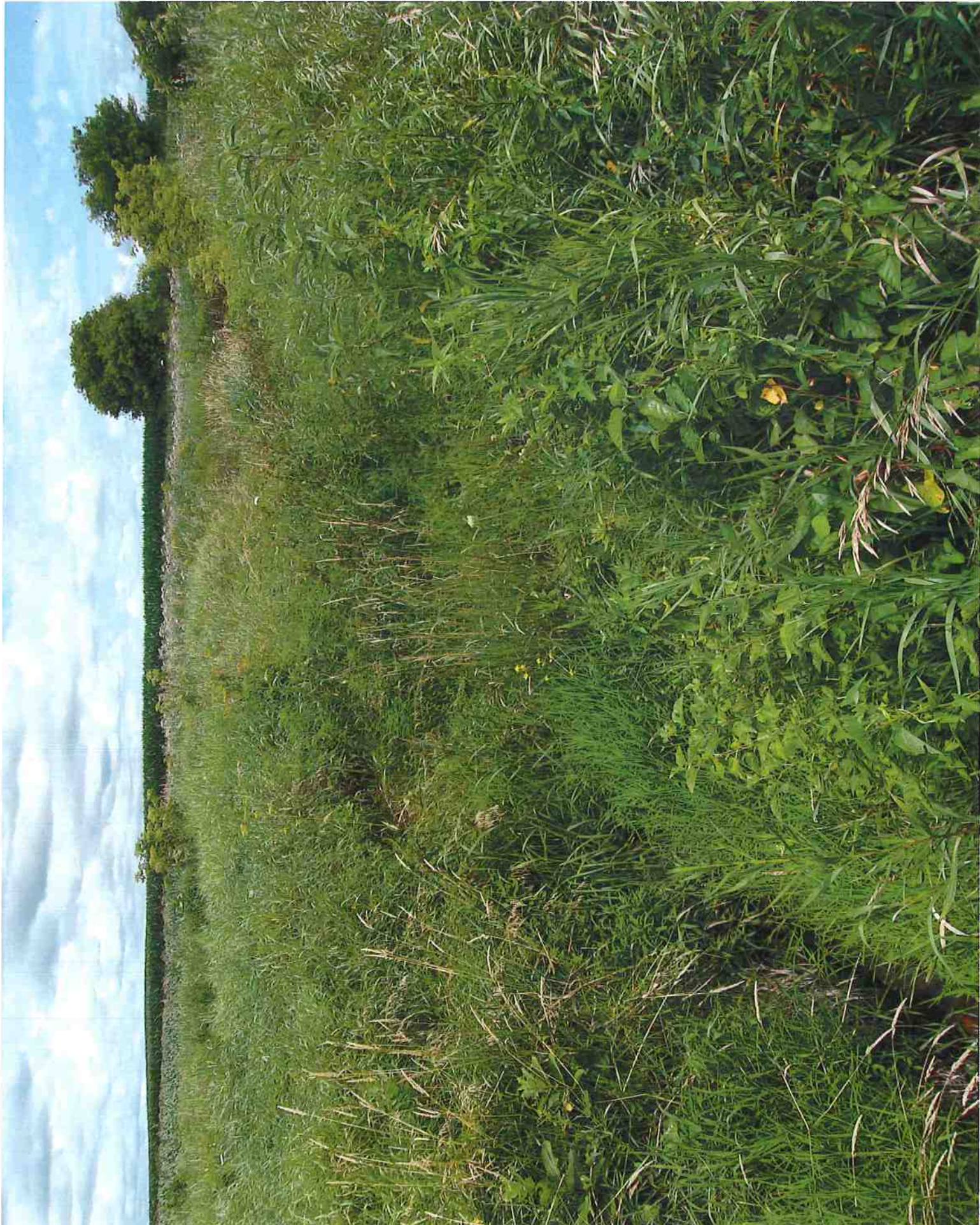
ERODED OUTLET TILE
