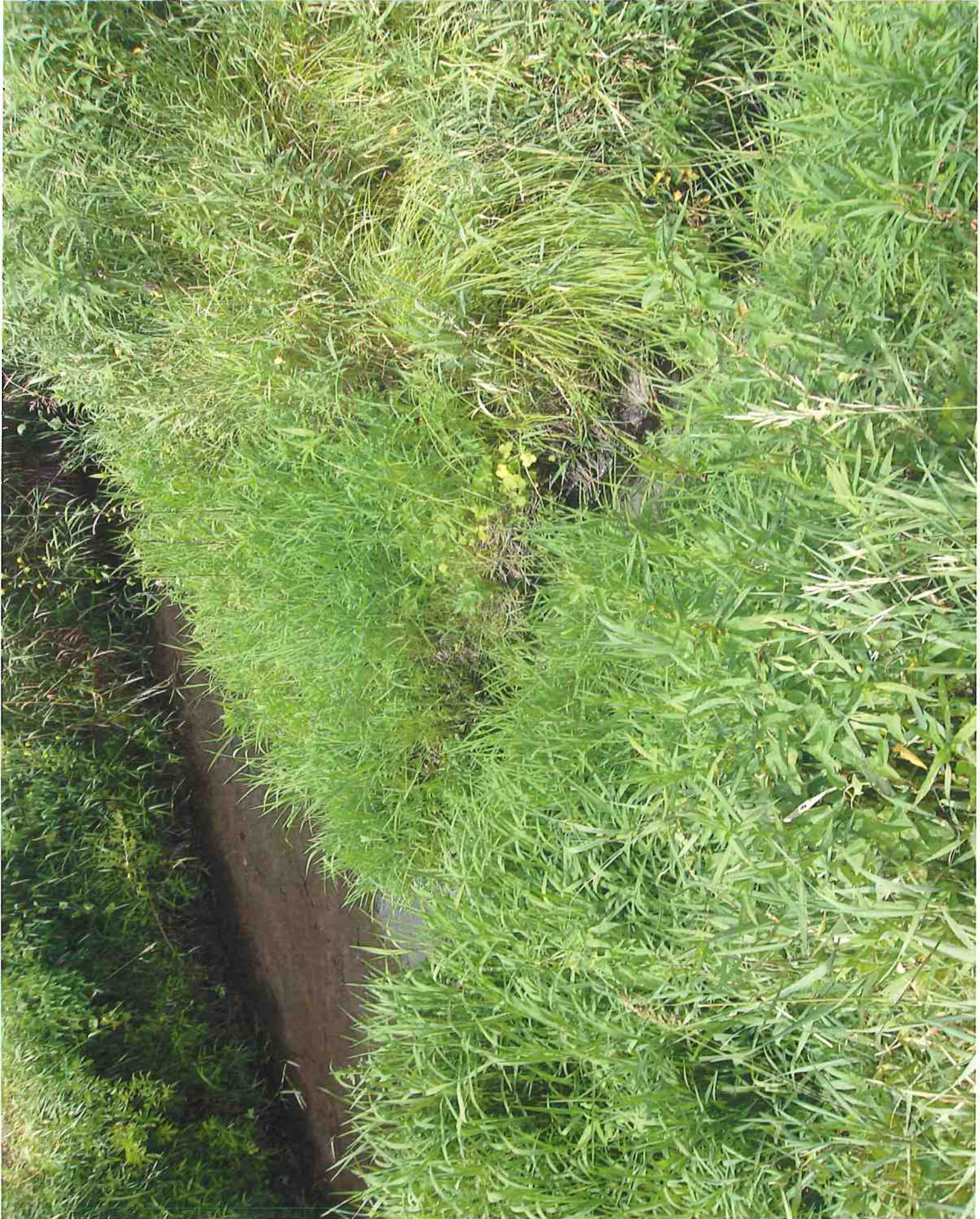
ERODED TILE OUTLET, 100' OF TILE MISSING
